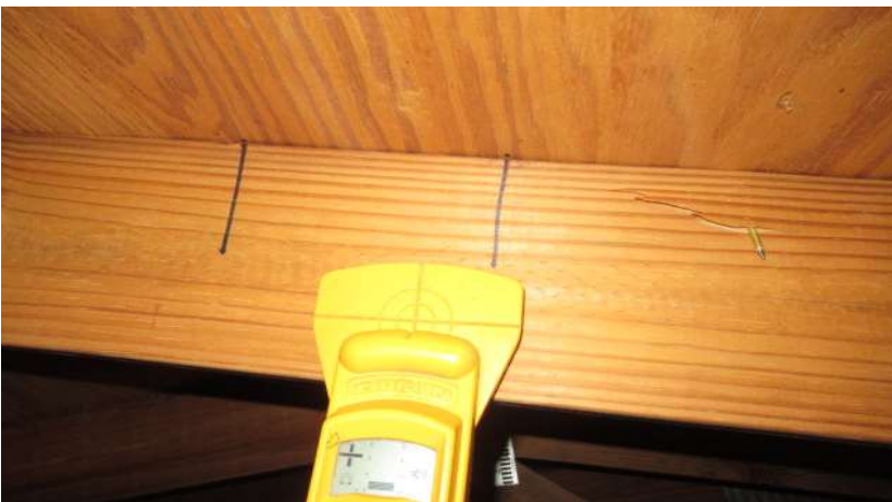
Nail location verified
