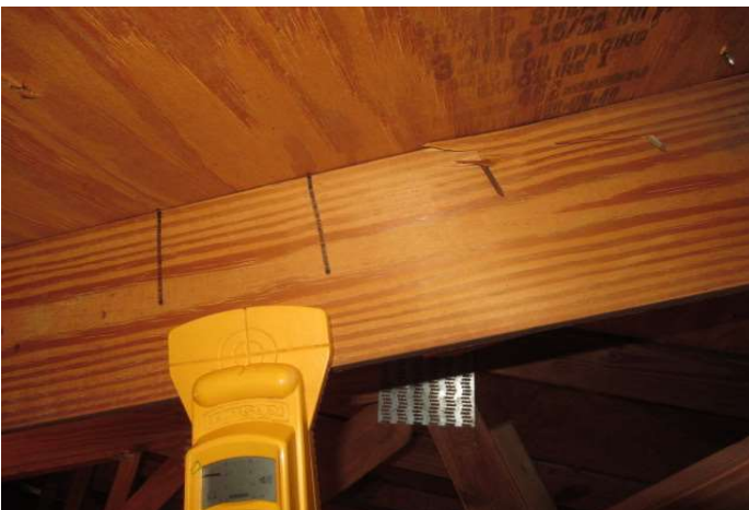
Nail location verified
