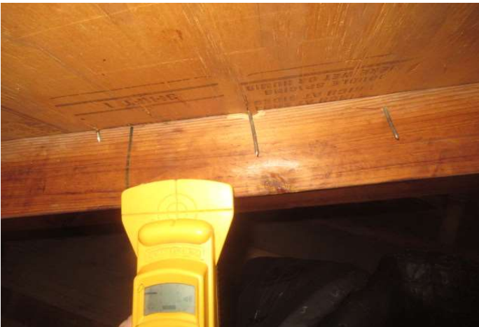
Nail location verified
